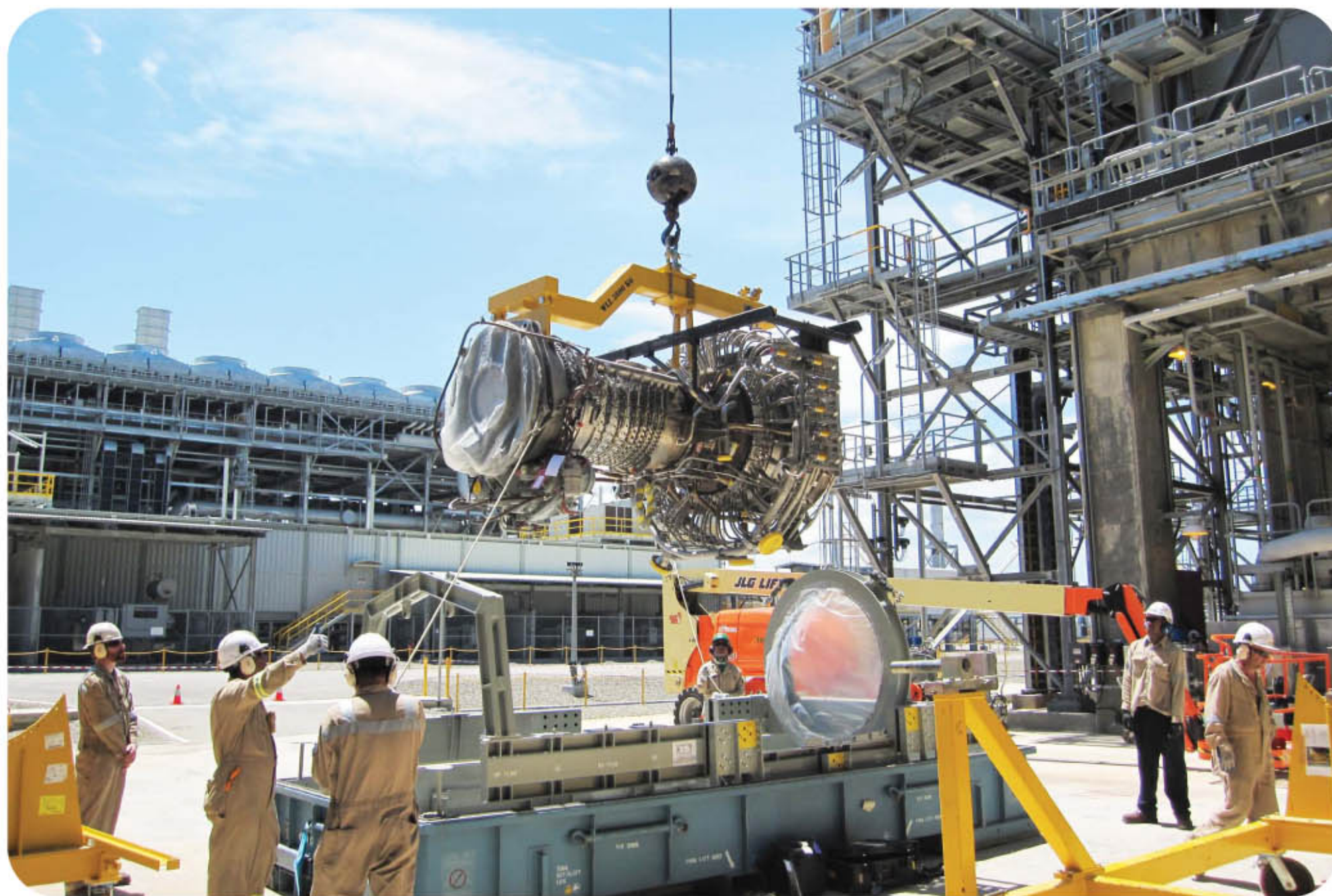
The new engine that was installed into the engine package during the maintenance work.
