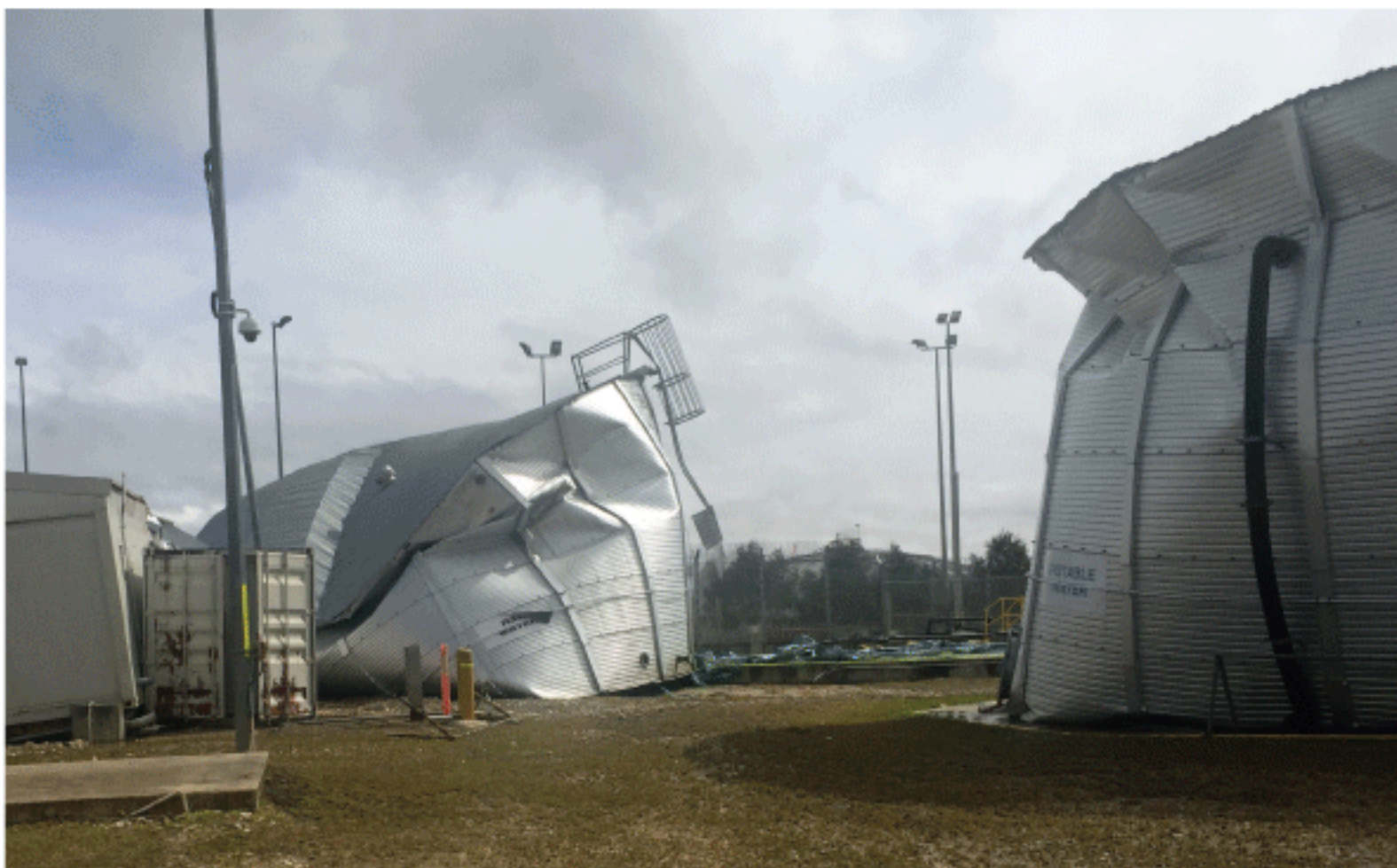
Water tanks at Hides Gas Conditioning Plant were damaged in the earthquake.
