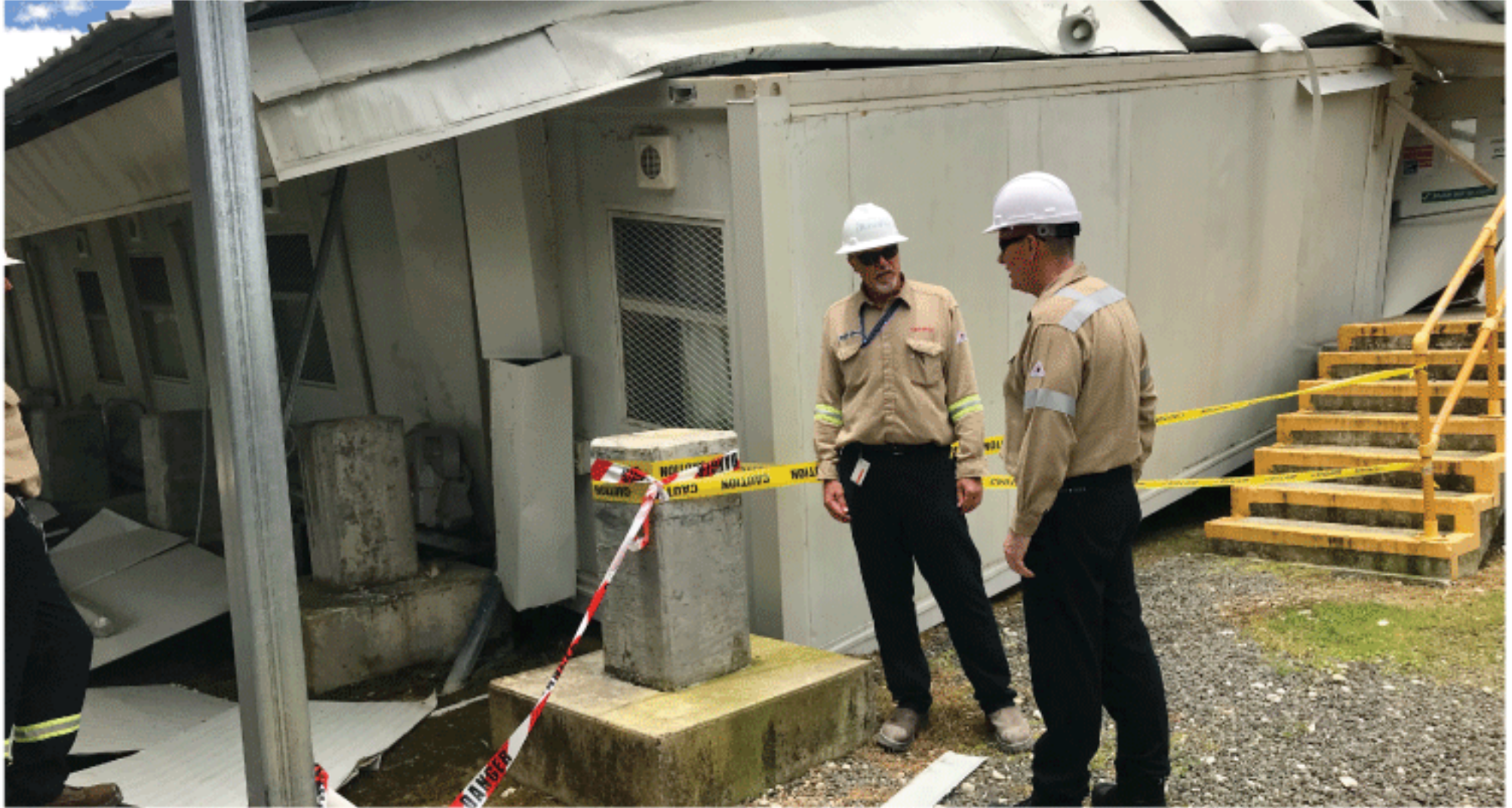
HGCP Senior Field Superintendent Murray Johnson (left) inspecting damage to buildings at HGCP with Executive Vice President Hugh Thompson.
