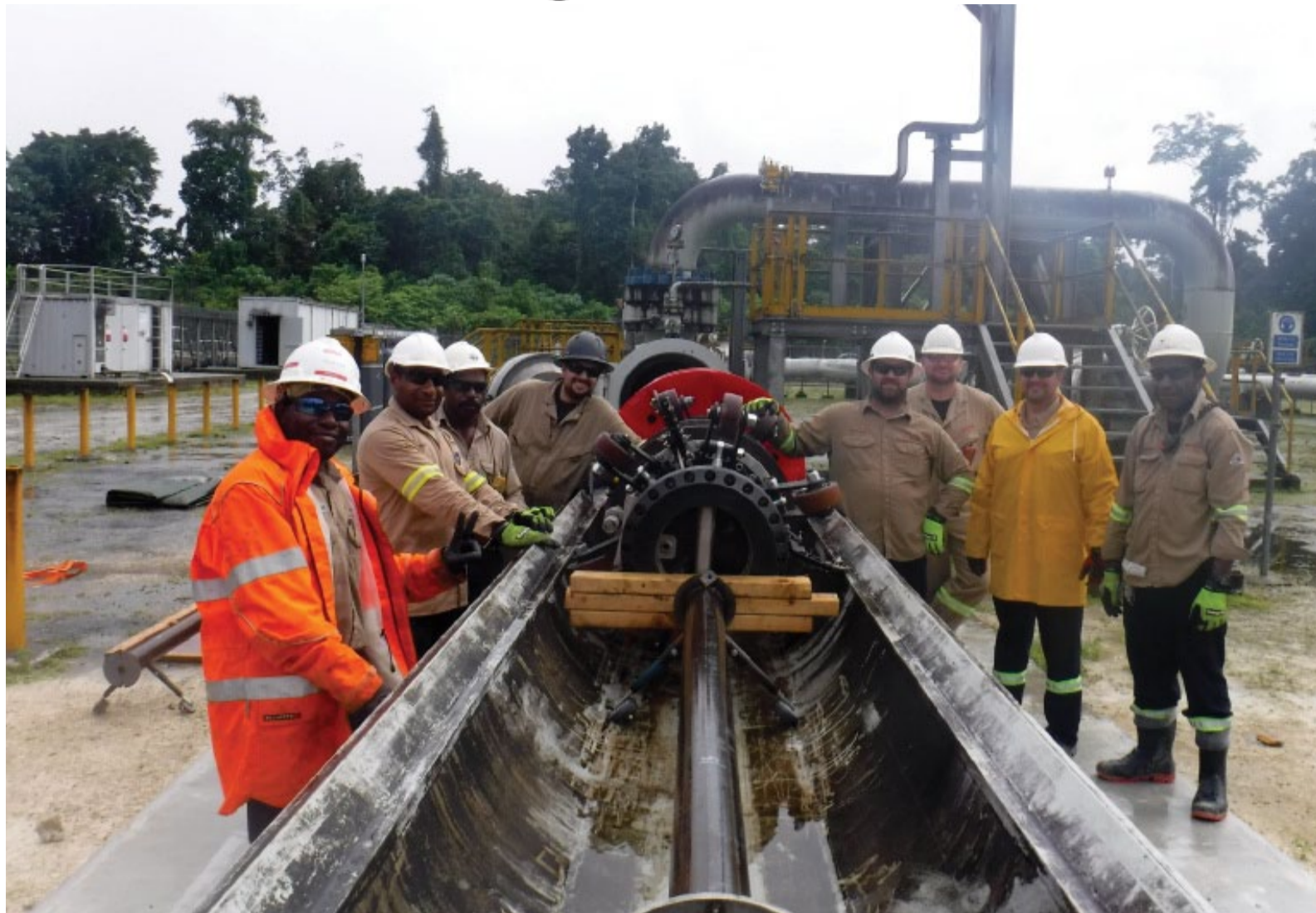
Maintenance crew launching the PIG at the Kopi Scrapper Station in Hela Province.
